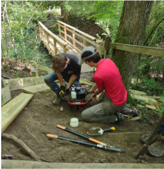
Student workers install steps on a trail in the Miami University Natural Areas. With nearly 1,000 acres and 17 miles of trails in our backyard, the Natural Areas are an invaluable resource for resilience, recreation, and research.
