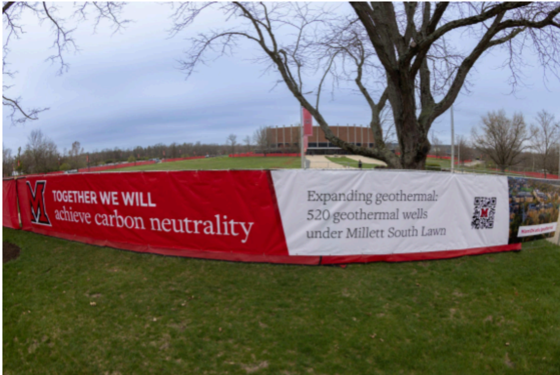
Construction fence banner for the North Geothermal Expansion project. 520 geothermal wells, 850 feet deep, will be drilled under the front lawn of Millett Hall starting this summer.
