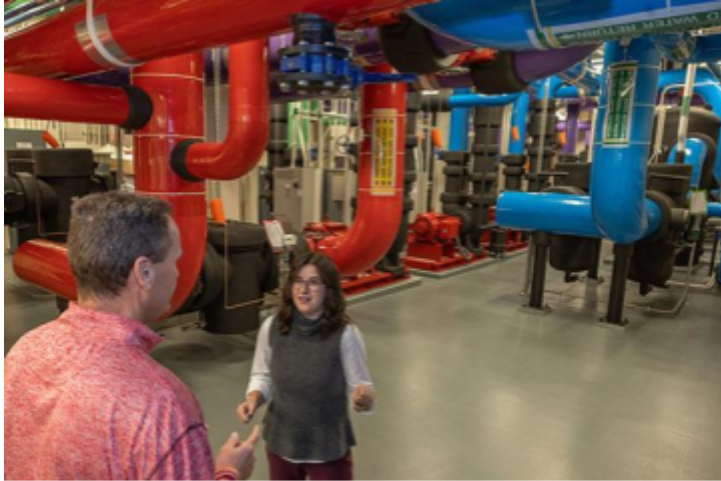
Inside the Western Geothermal Plant: Larry Davidson, Hydronics Operations Systems Manager, and Olivia Herron, Sustainability Director
